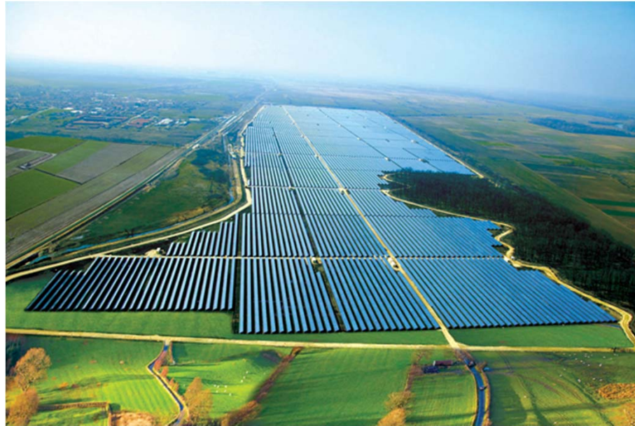
60.4-MWp Solar Power Plant in Bulgaria. (PRNewsFoto/SunEdison)
